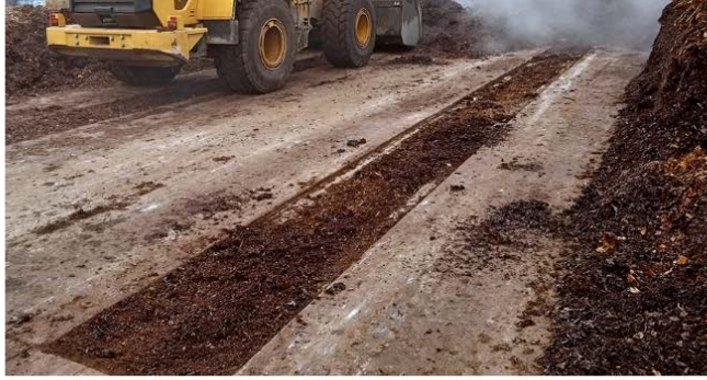
The 100 foot by 200 foot, 8 zone composting pad has pipes in the trenches of the aeration zones (above). The system runs in both positive and negative aeration modes.
