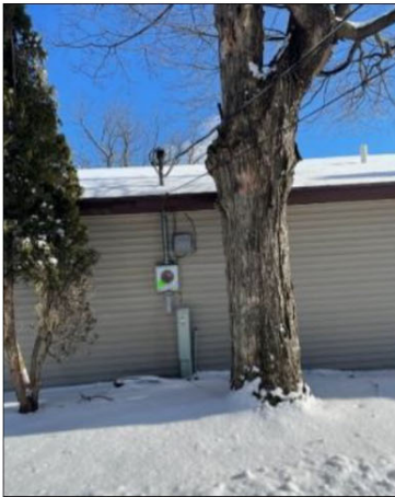
Approved overhead service, meter set only.
