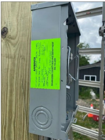
Meter socket inspection sticker.
