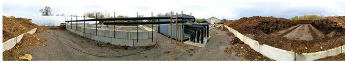
Panoramic view of Country Oaks Landscape Supply, showing, from left to right, the end of the composting pad, new greenhouse, biofilter, CAHR unit, the shop and sales building, and back to the composting pad and recessed channels. Photo by Jason McCune-Sanders, Agrilab Technologies Inc.
