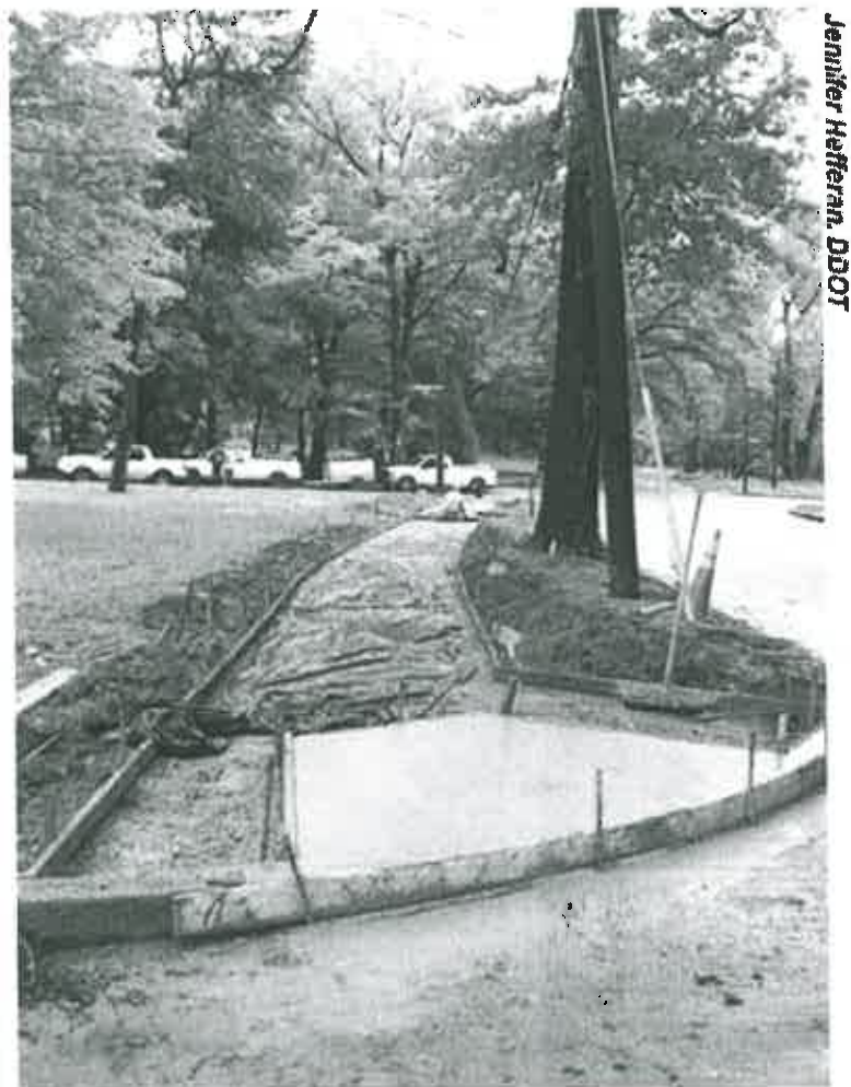
As part of the Safe Routes to School program, DDOT constructed segments of new sidewalk, such as this one, near Murch Elementary in Washington, DC.
