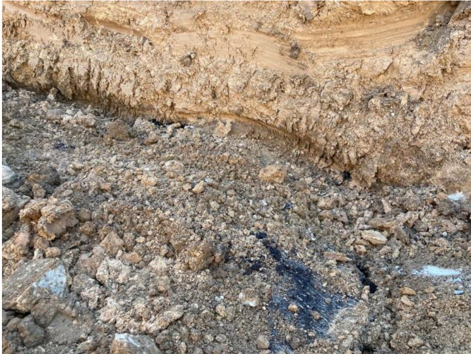
10/26/21- Chunks of asphalt discovered beneath the clay layer during the western side excavation at 5 feet (along the western wall of the excavated area, facing southwest)
