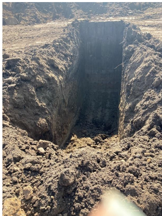
10/6/21 –Test Pit #4, approximately 8 feet deep (located on the northeast on the property)
