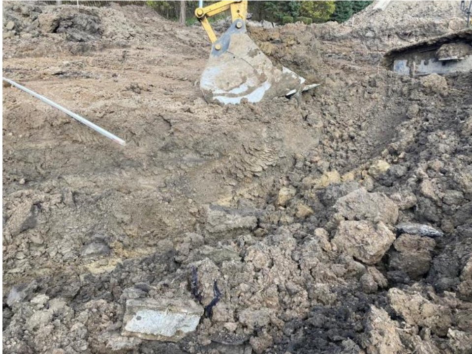
11/1/21- Fill material encountered to the depth of 14 feet in the center of the site (facing northeast)
