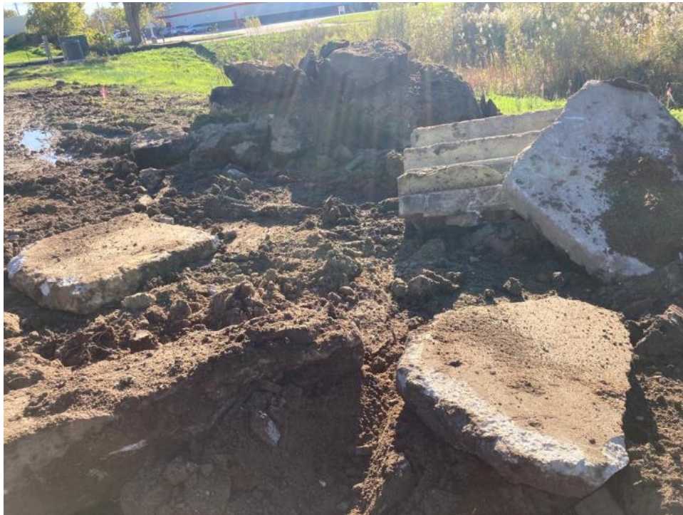
10/26/21- Chunks of asphalt and concrete excavated through western side excavation (facing southwest)
