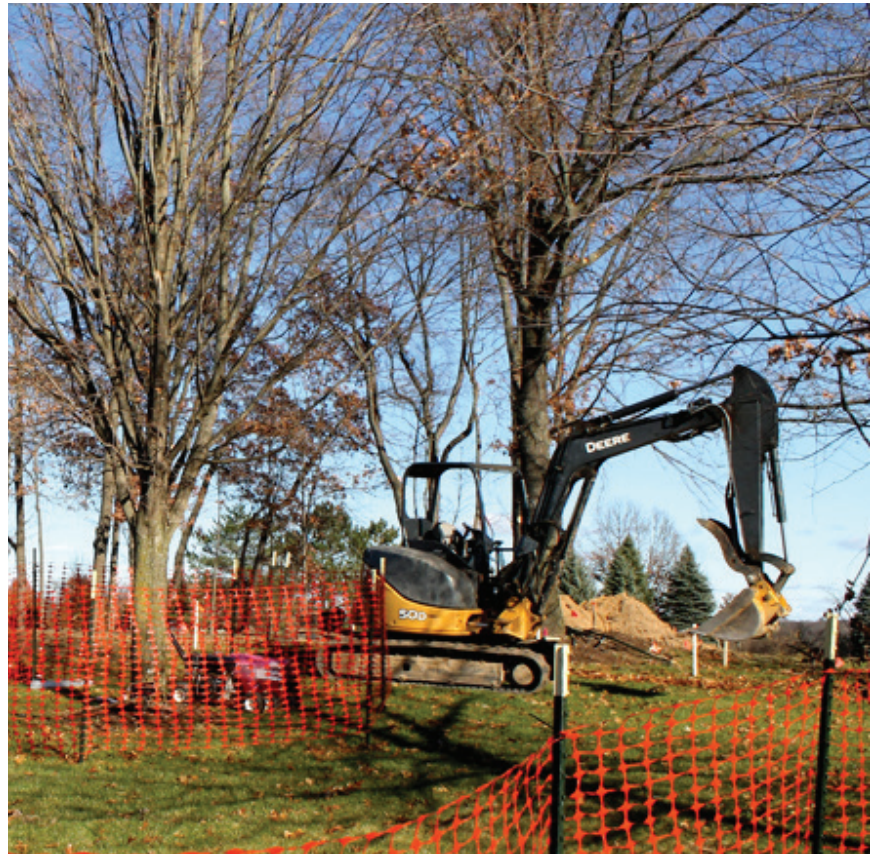
Construction began last month on the newly named Friendship Park – on the grounds of the Cascade library.
