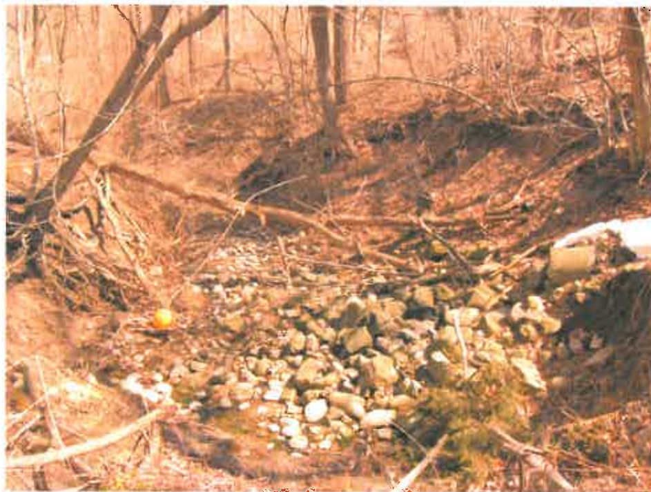
Unstable grade and eroding banks near Forest Hill Condominiums (stabilize channel and banks)
