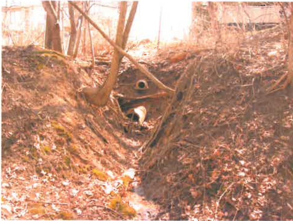
Typical eroding outfall structures (install drop structure and new outfall tile)
