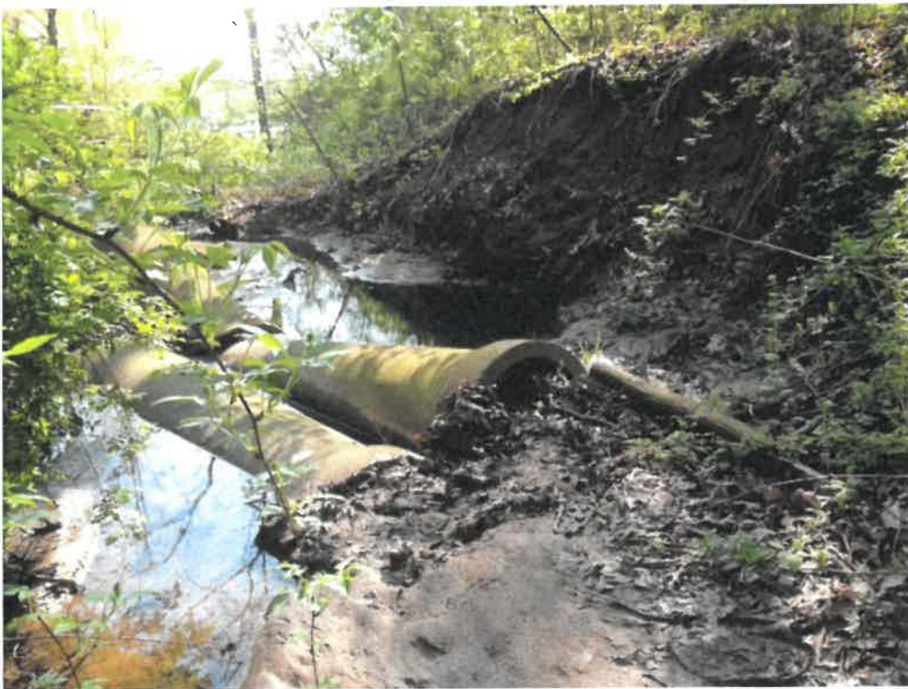
Dislodged storm pipes; erosion; sedimentation—Forest Creek District
