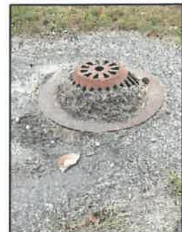
Plugged catch basin – district unknown
