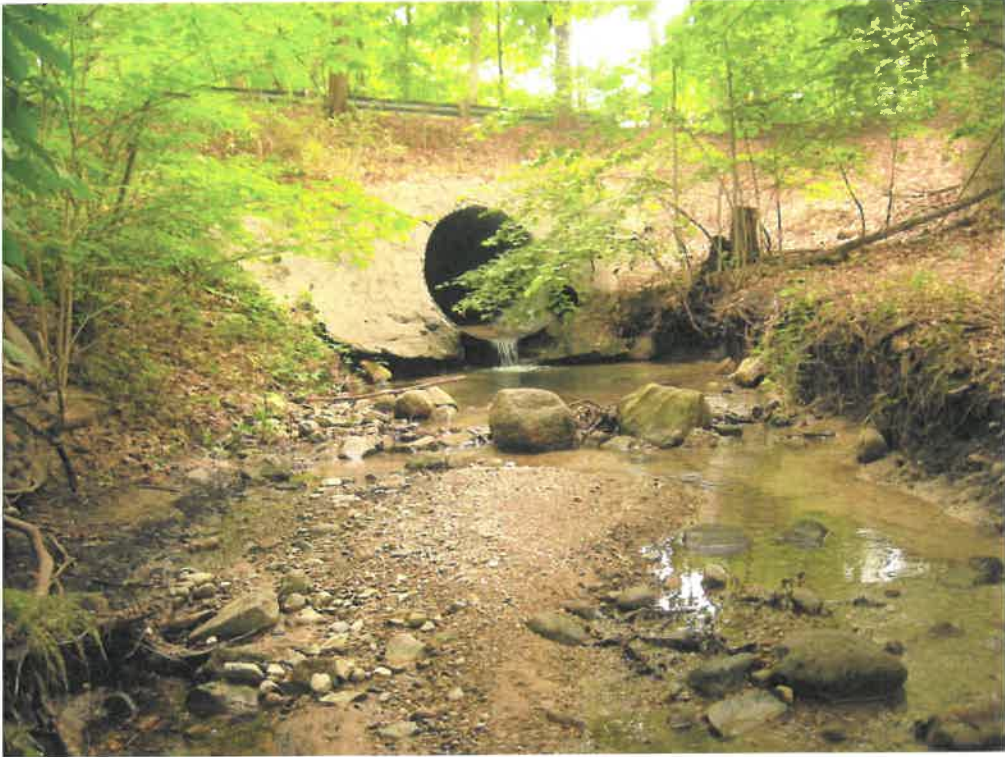
Perched culvert—Cascade Woods District
