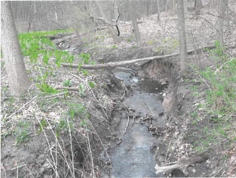
Channel headcut; erosion; poor floodplain connectivity; Hidden Hills District
