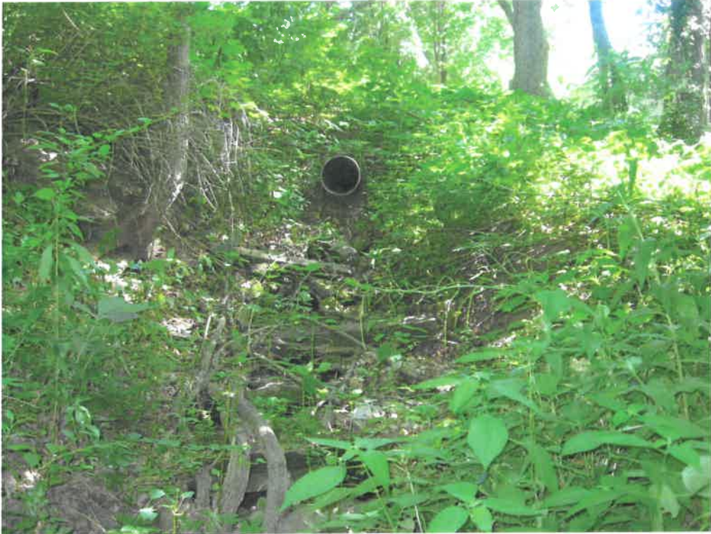
Eroding outfall; Quiggle Lake District
