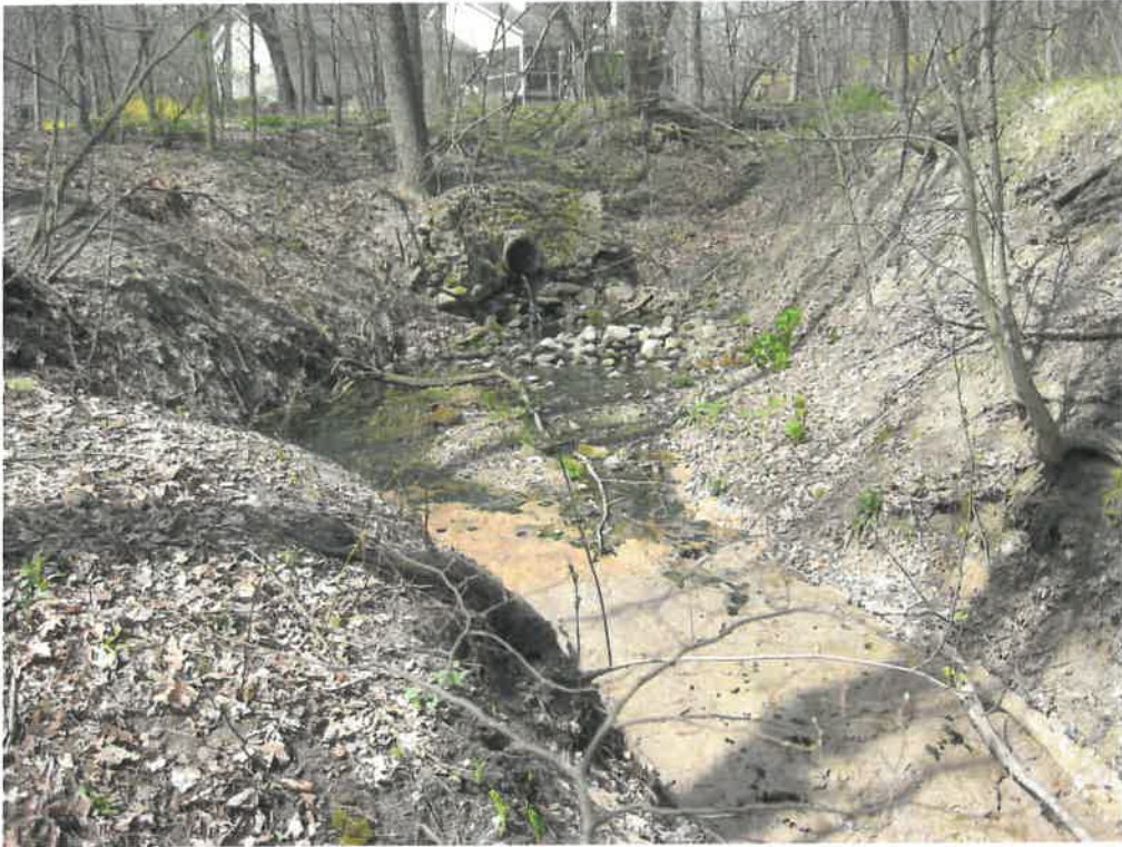
Storm outfall causing erosion in steep ravine —Tammarron District
