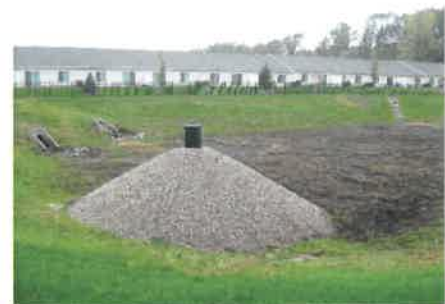
Private detention basin – Schoolhouse District
