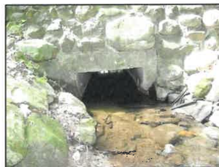
Private undersized culvert - Sturbridge District
