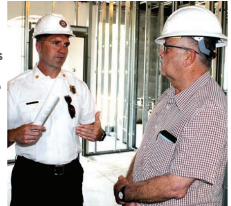
Cascade Township Fire Chief Adam Magers answers questions from Township Trustee John Shipley during a tour of the construction site in June 2023.
