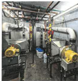
Heat exchangers and piping inside the AGT Compost Hot Box, 250-BR. Photo courtesy Agrilab Technologies, Inc.
