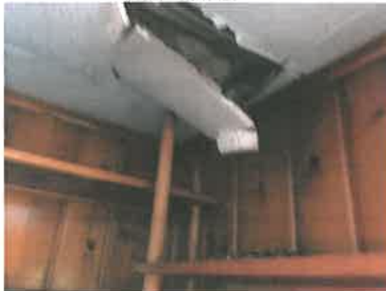
Evidence of water damage
