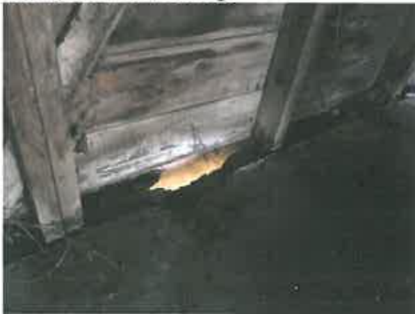
Holes / structural damage
