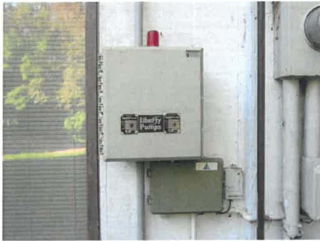
Liberty Pumps and sprinkling electronics
