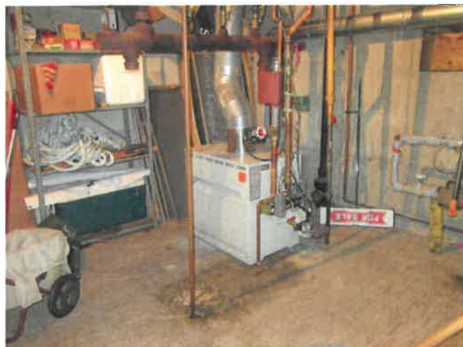
The mechanical room on the lower level
