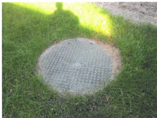
The Liberty Pumps manhole cover north of the building
