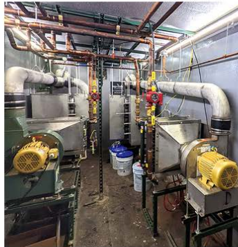
Heat exchangers and piping inside the AGT Compost Hot Box 250-8R. Photo courtesy Agrilab Technologies, Inc.
